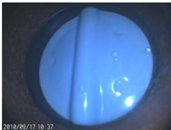
View of Valve from inside
