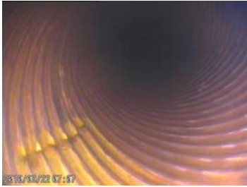
Straight View of Crack
